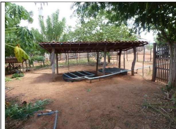
Figure 08 - Biological filters of the Family Bio-water System, with the pipes bringing the gray water from the house. 114
