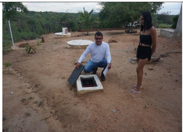
Figure 09 - Photo B - 3 parts of a RAC system: grease trap, filter and filtered water tank, in the background 115 .
