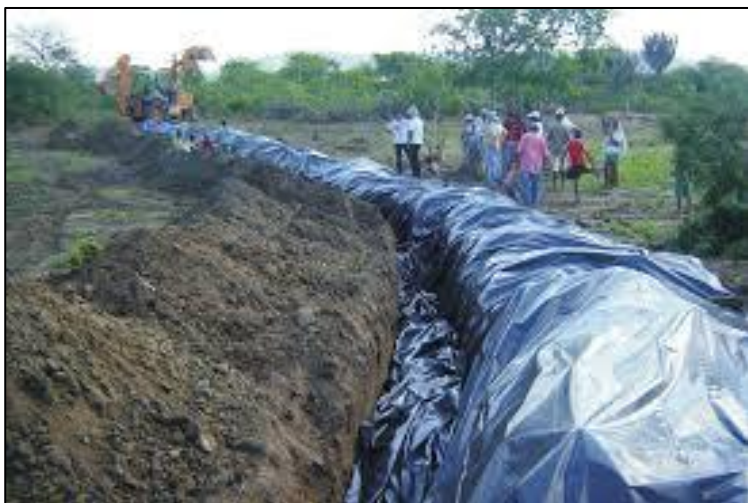
Figure 07 - Laying the waterproof tarpaulin of an underground dam under construction (MELO; ANJOS; SILVA; PEREIRA et al. , 2013)
