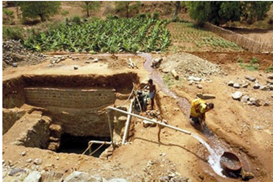
Picture 6: A view of the well where deepening and pipe-laying work is taking place.
