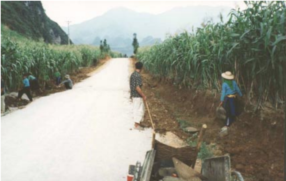
Agriculture Resources Conservation and Development Project in Quang Binh Province Rehabilitation of rural road.
