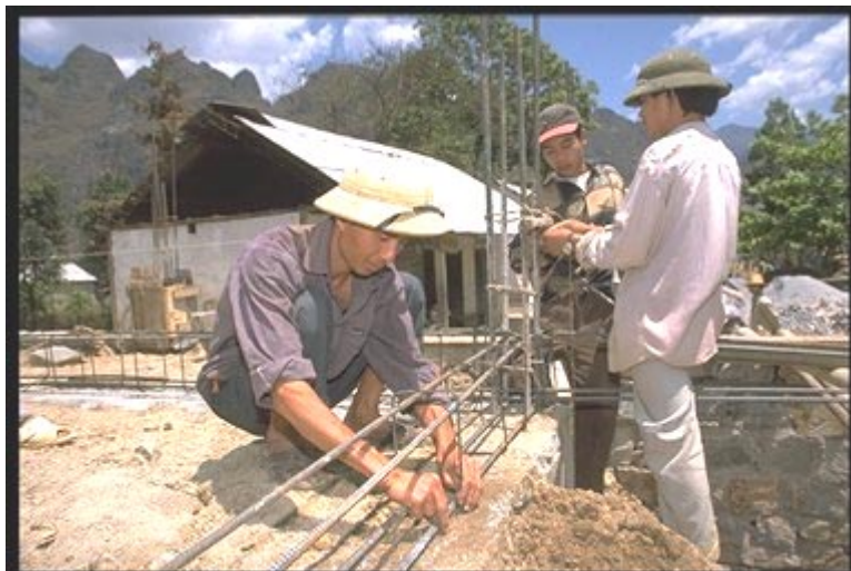
Ha Giang Development Project for Ethnic Minorities Construction workers build the project-funded district health centre in Yen Minh.
