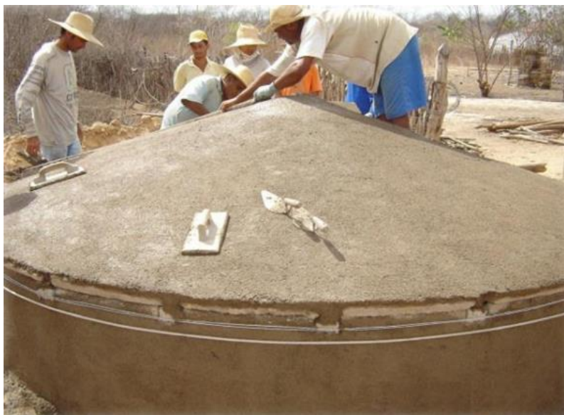
Figure 18: 16 thousand Liter Plate Cisterns - Cisterns Program 7
