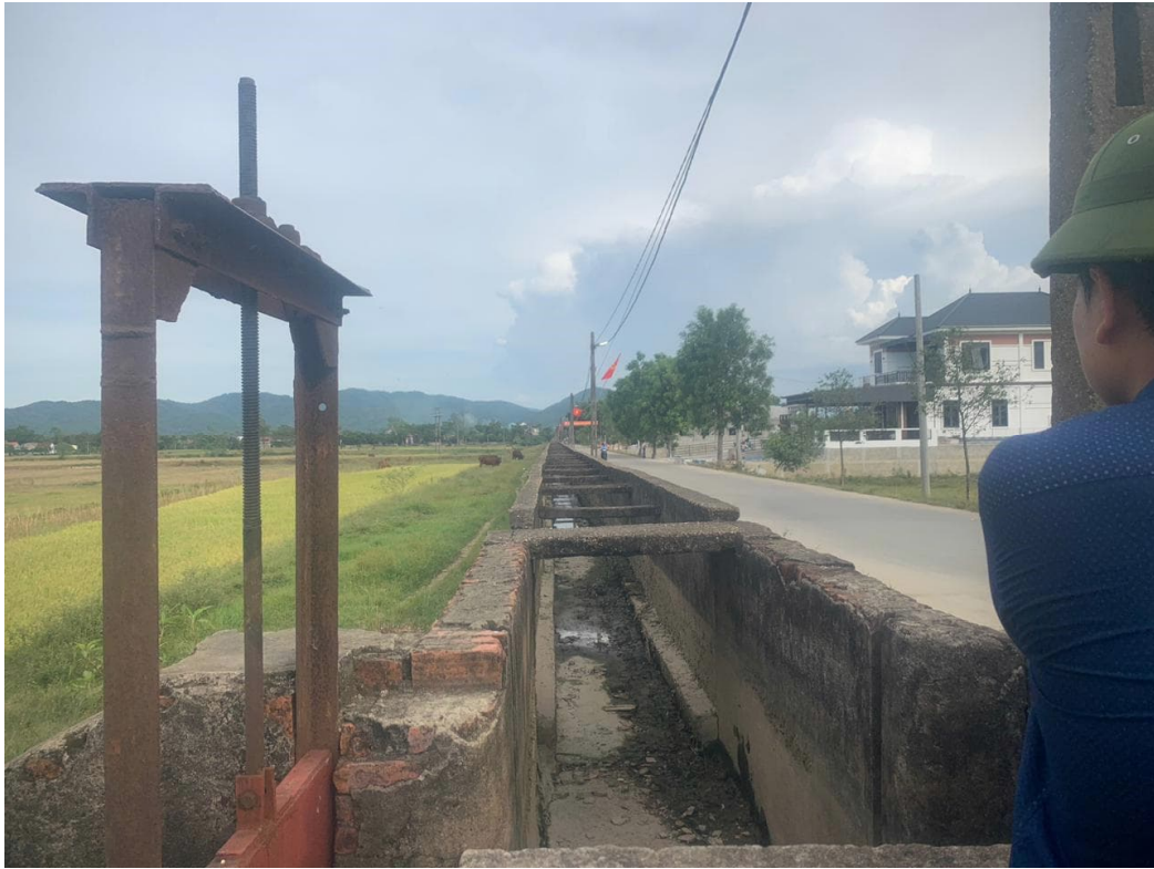
Irrigation canal adjacent to roads and farmers' fields that will be repaired
