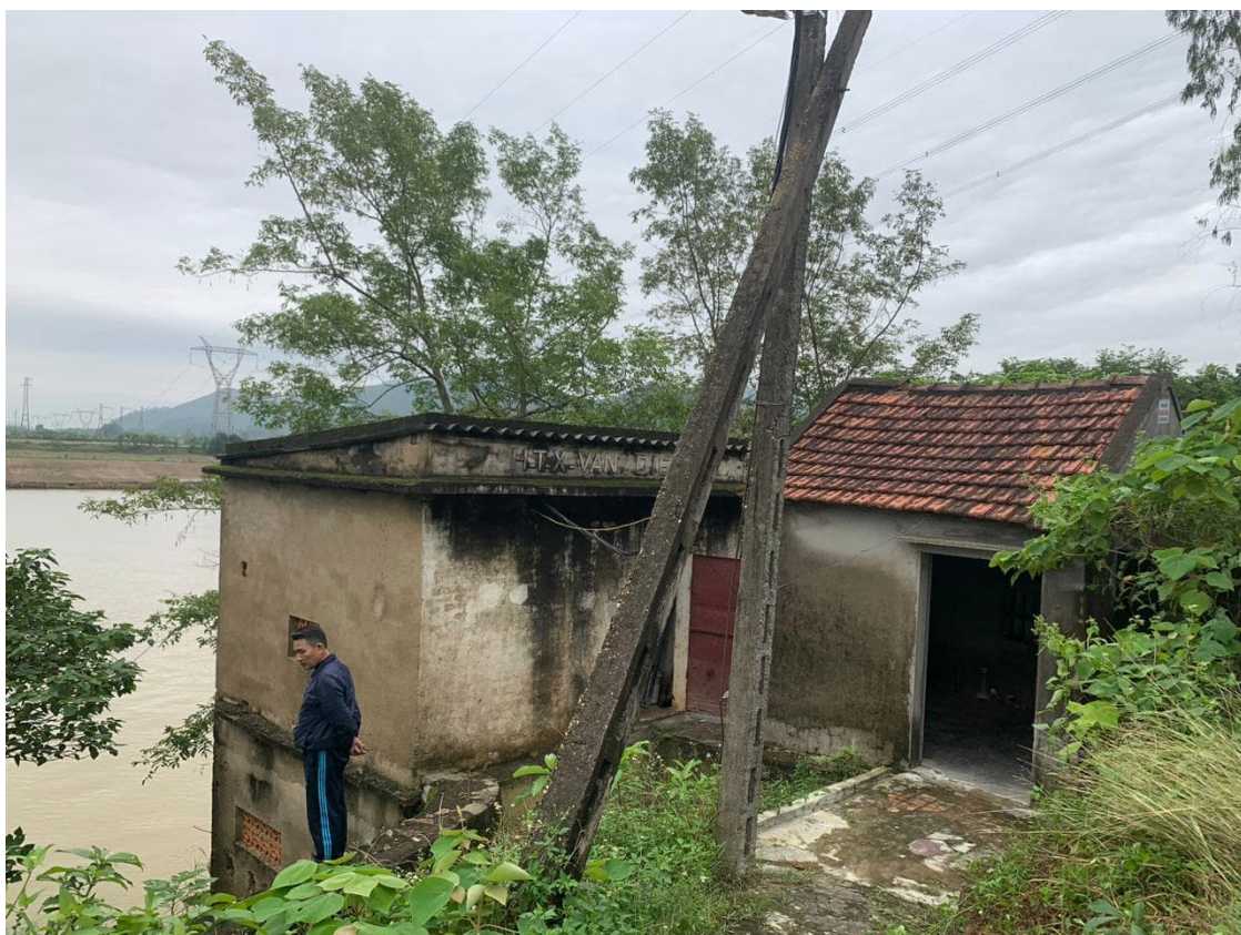
Community managed pumping station identified for upgrade in Nam Dan Town, Nam Dan District, Nghe An
